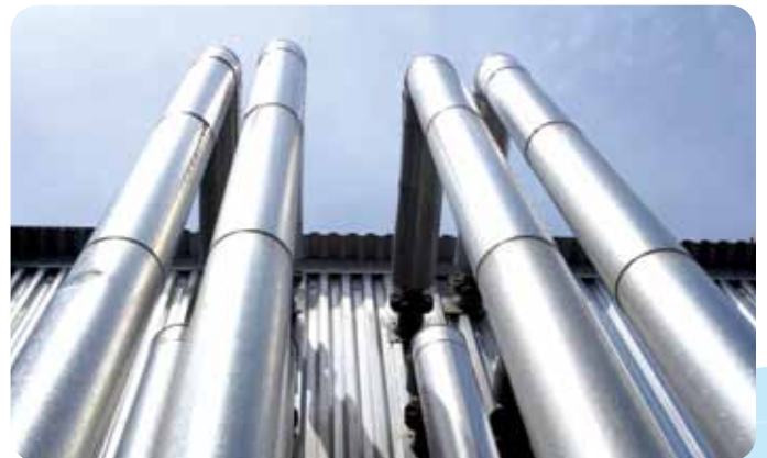
Silver Fern Farms’ Finegand meat processing plant in Balclutha is turning sludge from waste water into a valuable biofuel, reducing the company’s CO 2 emissions by 9,500 tonnes per year. The company aims for best practice in environmental stewardship and industry innovation.
